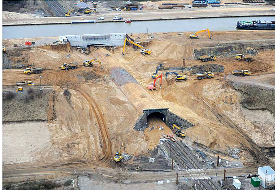
Bild 13 Abbruch Tunneldecke in zweiwöchiger Sperrpause der Bahn Demolition of tunnel soffit during a two weeks rail shutdown
